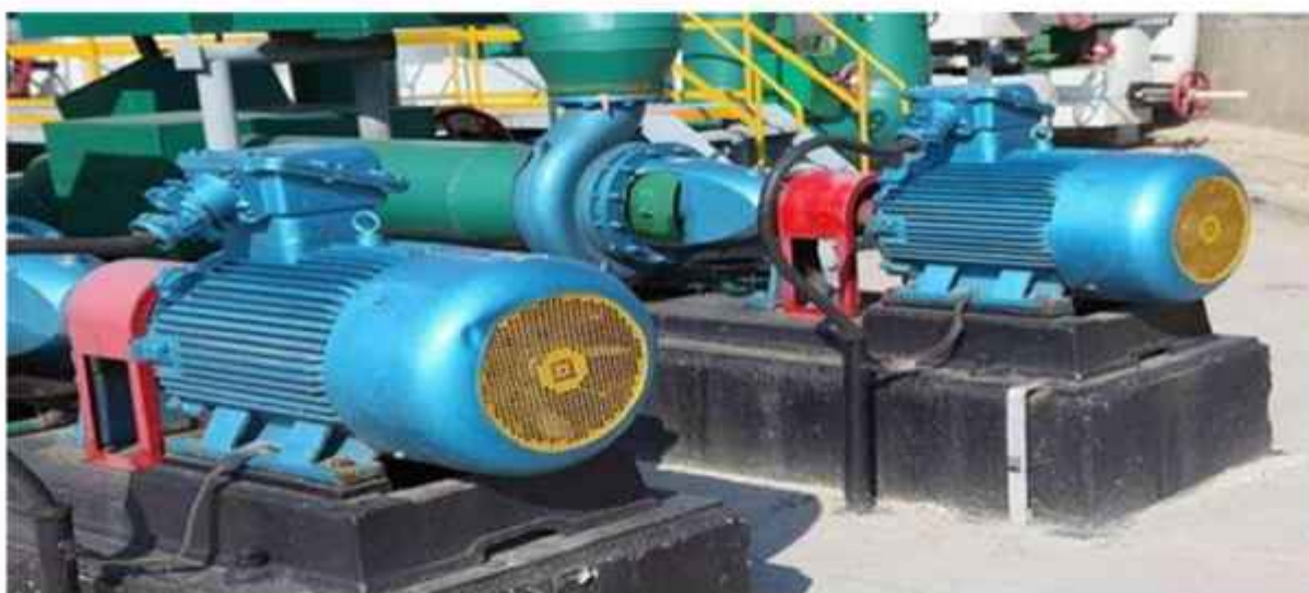
Pump House with IE3 Motor at SECL
