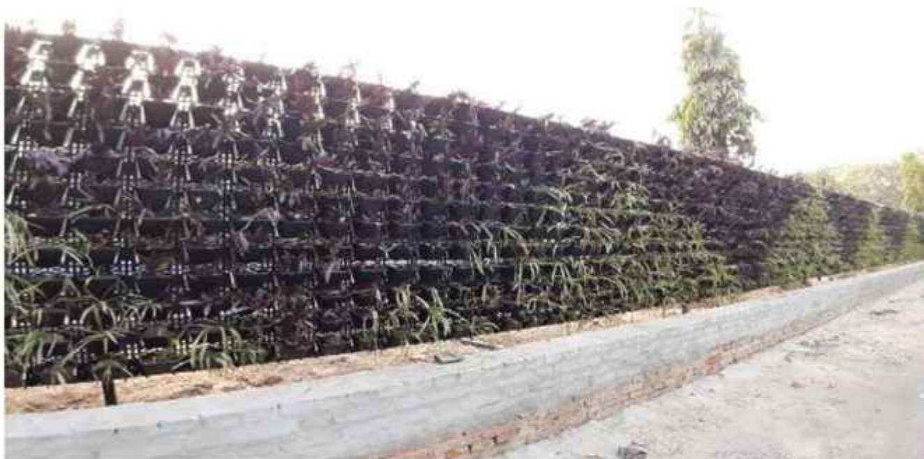
Vertical Greenery System in Basundhara Area, MCL
